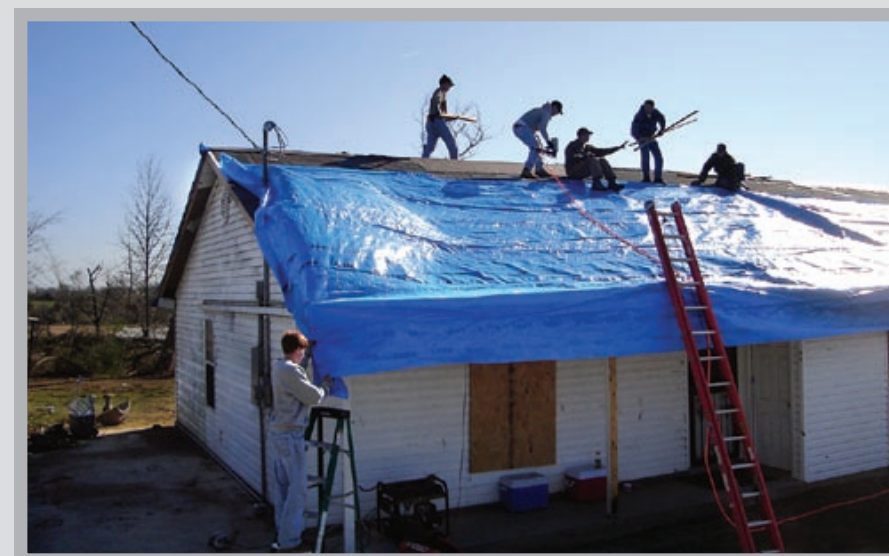
Calvary Chapel volunteers attach a tarp to a roof to keep out water and wind damage after a tornado destroyed several homes in Jackson, TN.
